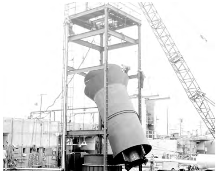
Figure 21: (Above) Construction of the Silo Model. The launch duct and exhaust ducts were installed in one piece. Courtesy R. Pickford.
