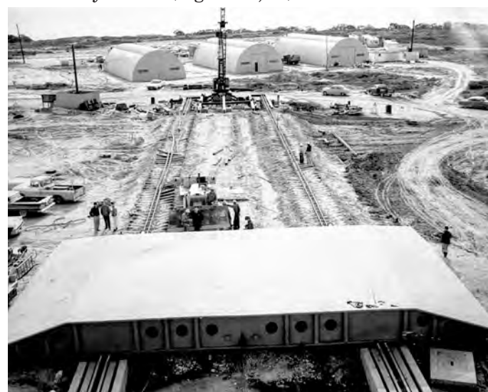
Figure 27: Silo Closure Door at Launch Facility 395-B, Vandenberg Air Force Base. The silo closure door was assembled as close to the launch duct as feasible. Here the door is being moved to Site 395-B. Author's Collection.
