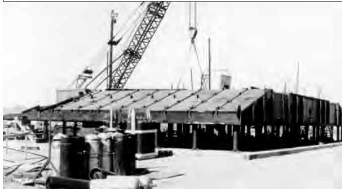
Figure 26: Silo Closure Door Detail. Upper: Diagram illustrating the “eggcrate” construction of the massive 700-ton silo closure door. The top and bottom plating was 3.5-inch battleship armor. The interior webbing supports varied from 1.375 inches to 2.5 inches in thickness. Lower: The silo closure door was prefabricated in sections and assembled on site. The pedestals will be removed and the door lowered onto temporary rails for movement onto the silo. Courtesy Titan Missile Museum Archive.
